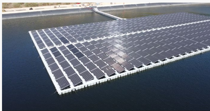
Floating photovoltaic installation in Guaro, Málaga, Spain, by the firm Landatu Solar. Photo: Landatu Solar
